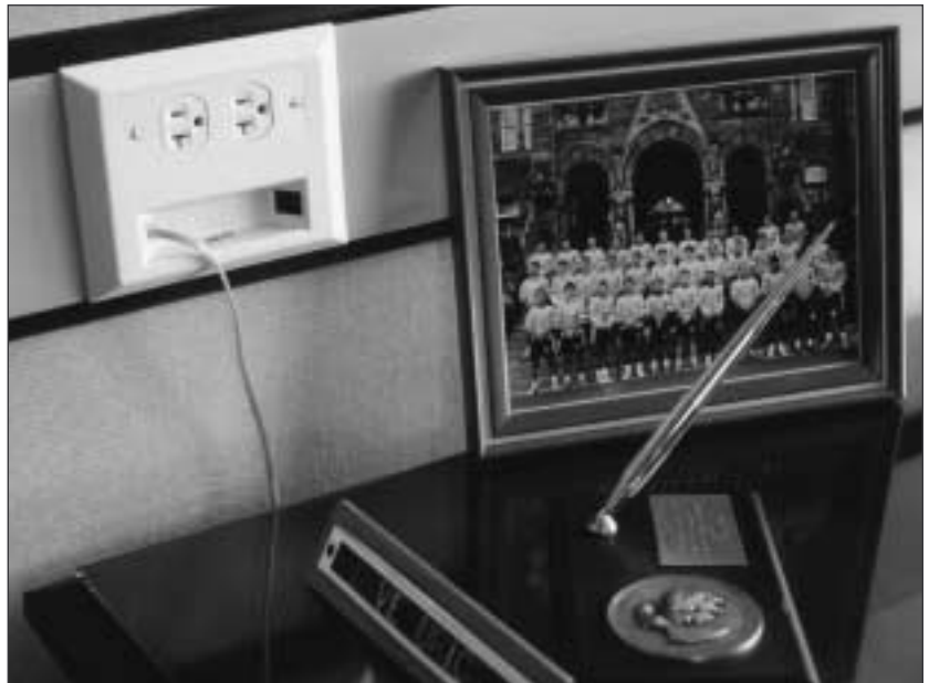
Access 5000 Raceway installed at chair rail height.
