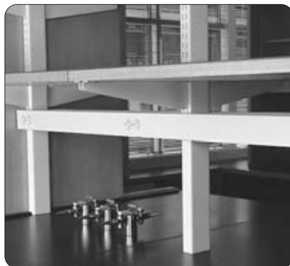
3000 Series raceway used in a lab installation.
