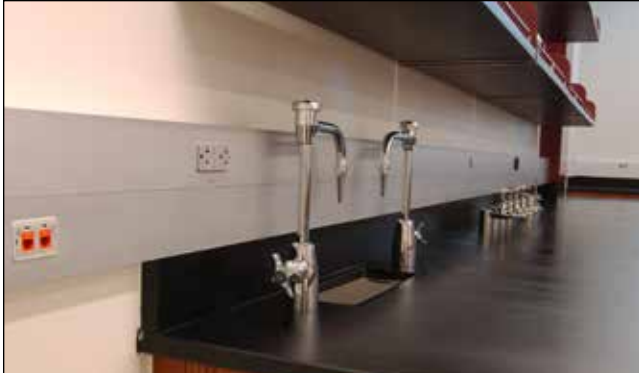
An ALA4800 Series Raceway installation in a laboratory is both functional and aesthetically pleasing.
