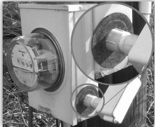
Traditional Application which compromises the enclosure's 3R rating
