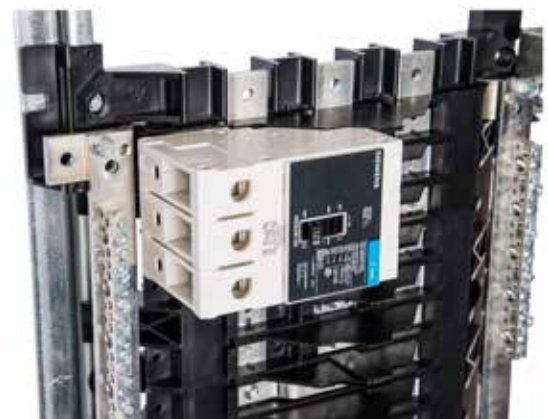
Example of Back-fed NGB Main breaker installed
