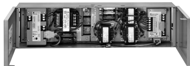
Voltage Module Interior View
