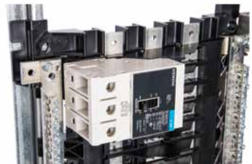
Example of Back-fed NGB Main breaker installed
