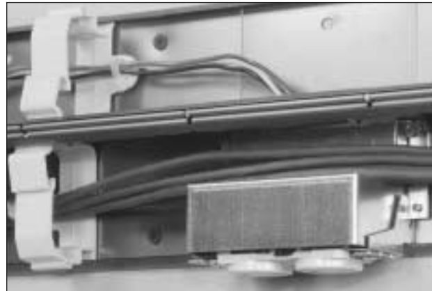
Communication cables can now safely transition over power device.
