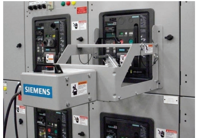
Remote Racking Device
