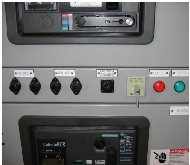
Control port on WL Switchgear
