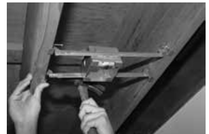
Step 3: Nail or screw to wood joist and adjust unit vertically or horizontally to ensure flush alignment
