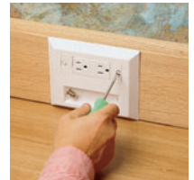
Install covers and receptacle plates. Complete the installation with voice and coax connectors.
