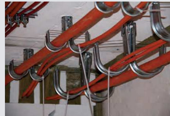
J-Hooks and cables in fire chamber before fire test
